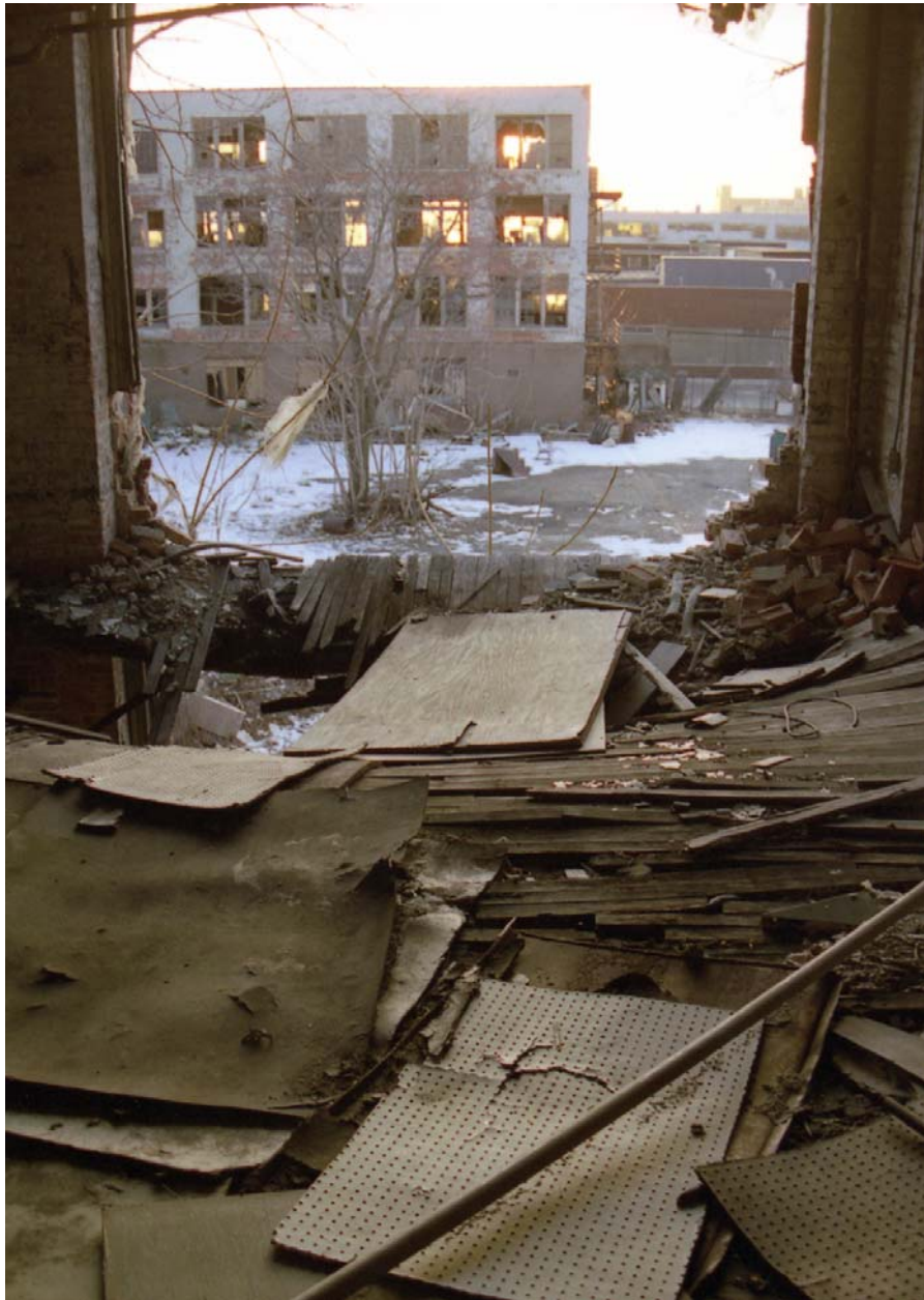
With this improvised ramp behind a demolished wall, a scrapper has created an exit from the Studebaker Corporation complex.
