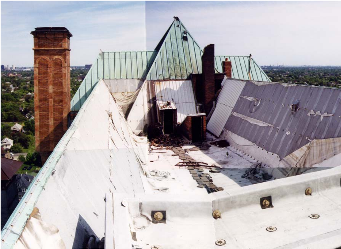
Stripped copper roof of the Lee Plaza high-rise.
